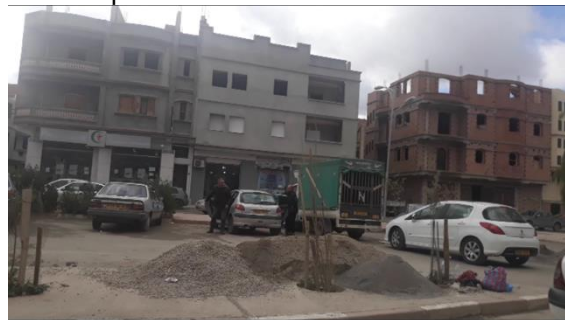
Fig. 5– Construction of new multi-storey houses after demolition of old ones. Rental for residence, professional and commercial activity.
