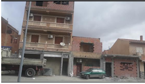
Fig. 6 – A renovated house on the right and construction of another floor for the house on the left.
