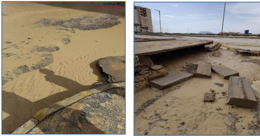
Figure 07: Damage to public spaces caused by floods in Tebessa.
