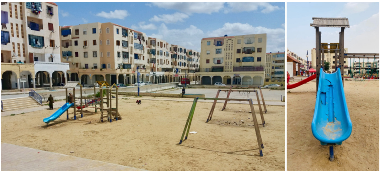
Figure 43 The damaged play structures of the neighborhood of 420 housing units (Source: Author).
