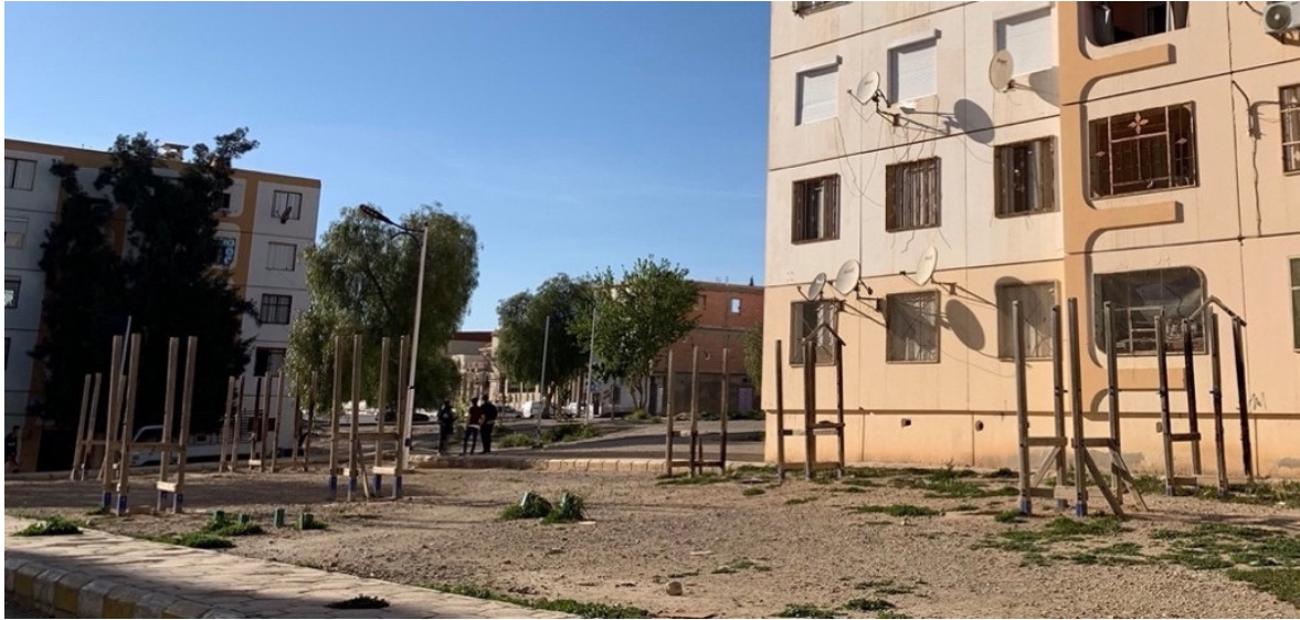
Figure 44 The damaged play structures of the neighborhood of 1500 housing units (Source: Author).
